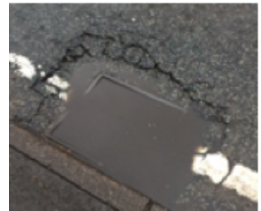
Village road gullies collapsing from the weight of the large vehicles.
