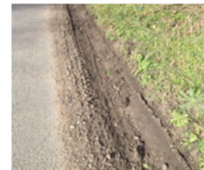
The lorries have damaged the verges on all of Hunsdon's roads.
